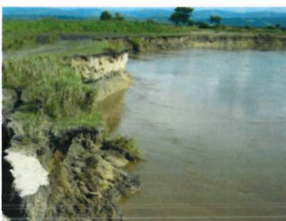
Plate 4.6: Loose soil at River Semliki banks
