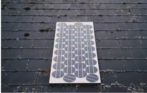
Figure2- 11: shows a solar panel fixed on a roof
